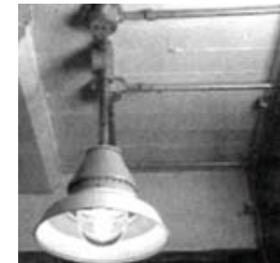
Typical Class 1 Div 1 conduit installation
