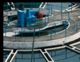
Waste Water Treatment Plants
